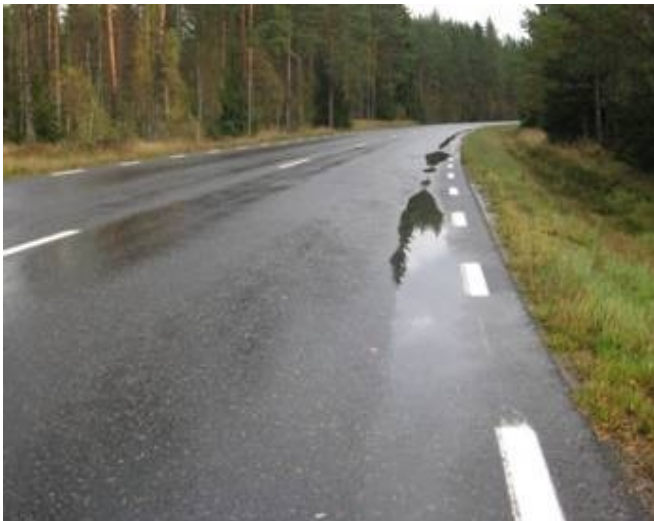
Rutting (plastic deform.)
