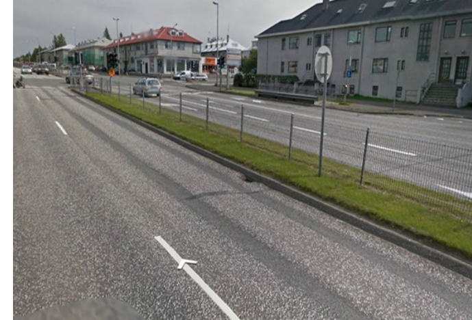
Abrasion (studded tyre wear)
