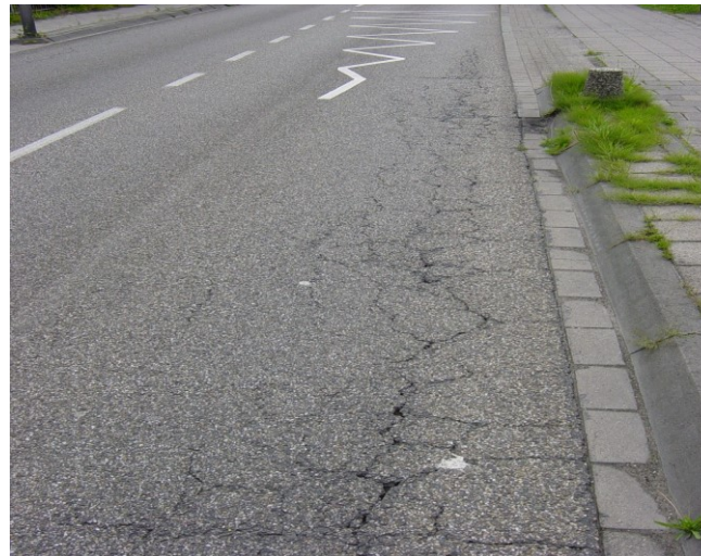
Fatigue cracking (bottom-up)
