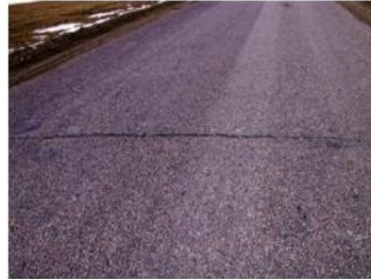
Tversgående sprekker Travers cracking
