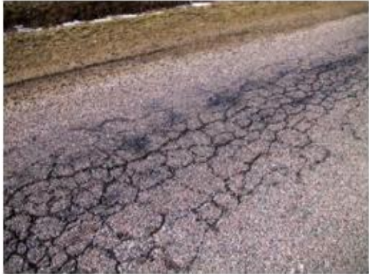
Krakelering Network cracking
