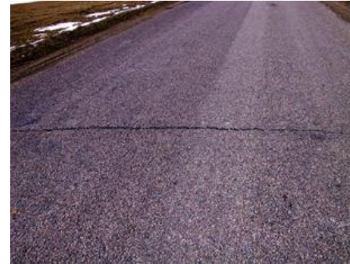
Tversgående sprekker Travers cracking
