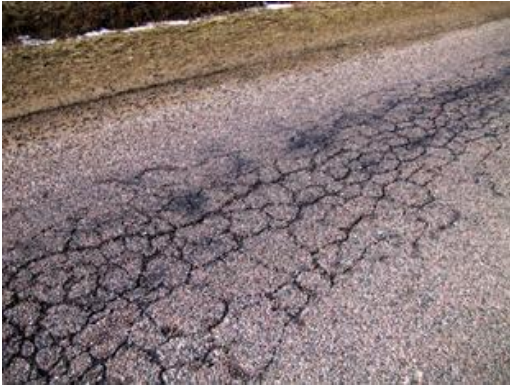
Krakelering Network cracking
